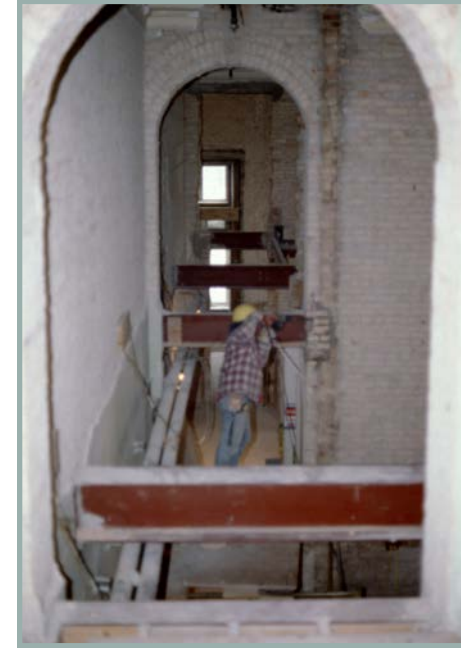
A construction worker removes a beam from the overfloor, or mezzanine, that once subdivided the south corridor near the Lieutenant Governor's Office.
